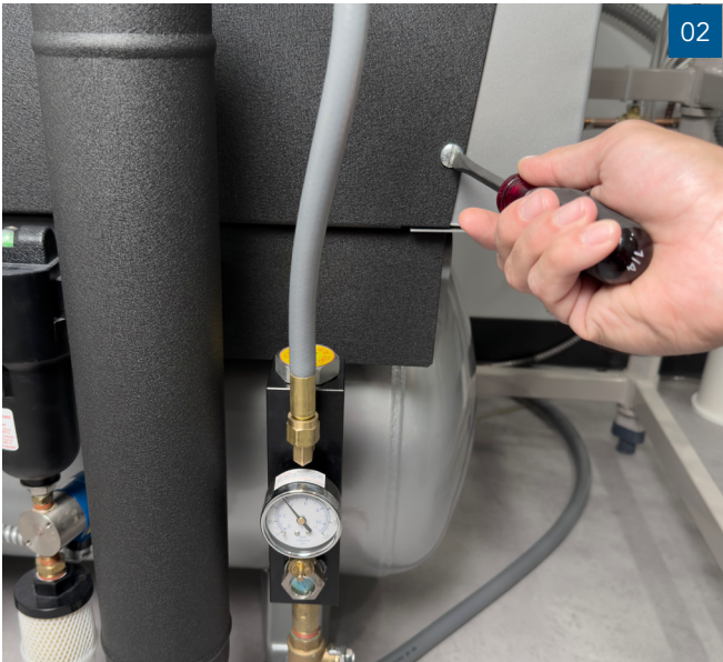
02 Final touches help confirm your equipment is operating properly before we leave your facility.
