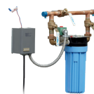
Water Filter Bypass
